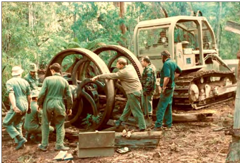
Army Reserve personnel removing the fly wheels from the Crossley engine, while a bulldozer waits on. Photo: Ian Martin, 1988.
