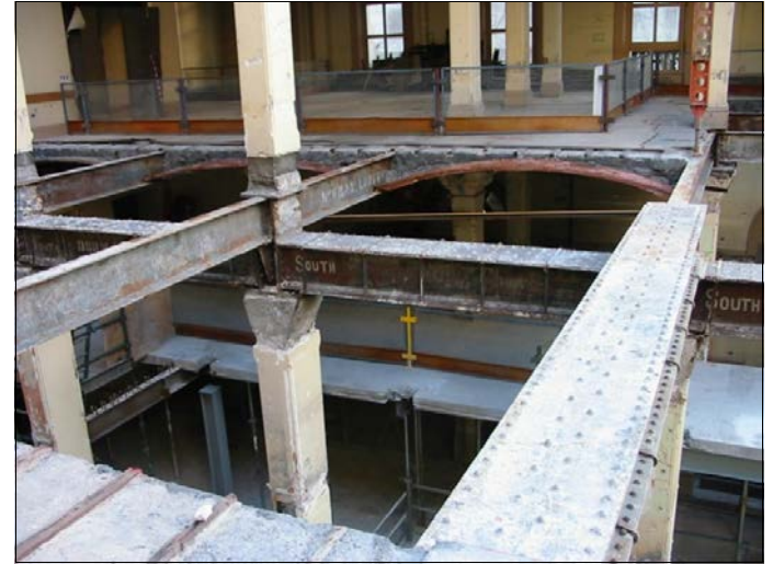
Melbourne General Post Office, Bourke & Elizabeth Sts, 1885-90 top floor extension. This view shows the floor structure, with Traegerwellblech flooring cut out. Photo: Miles Lewis.
