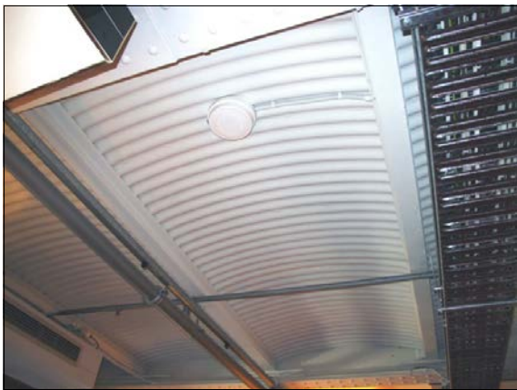
Verdon wing of the State Library of Victoria, 1886, Traegerwellblech flooring seen from underneath: Photo: Miles Lewis.
