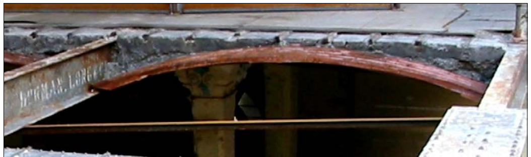
Detail of the top floor of the Melbourne GPO building, with a surviving red, rusty section of a Traegerwellblech arch, with one end resting on a Dorman Long joist and the remains of the concrete infill & floor sheeting above it. Photo: Miles Lewis
