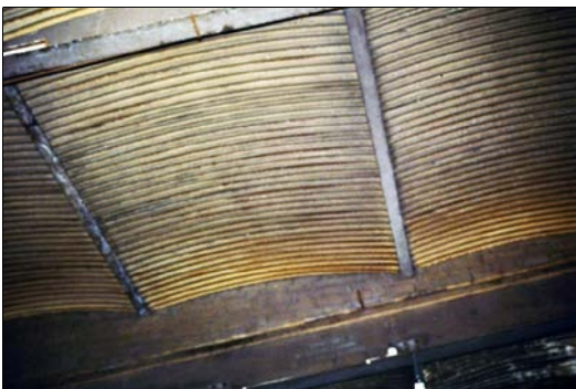
New Zealand Loan & Mercantile Agency Wool Store, off Tennyson St, Kensington, Melbourne, extension by Oakden & Ballantyne, 1910, floor of linking bridge from below. Photo: Miles Lewis.
