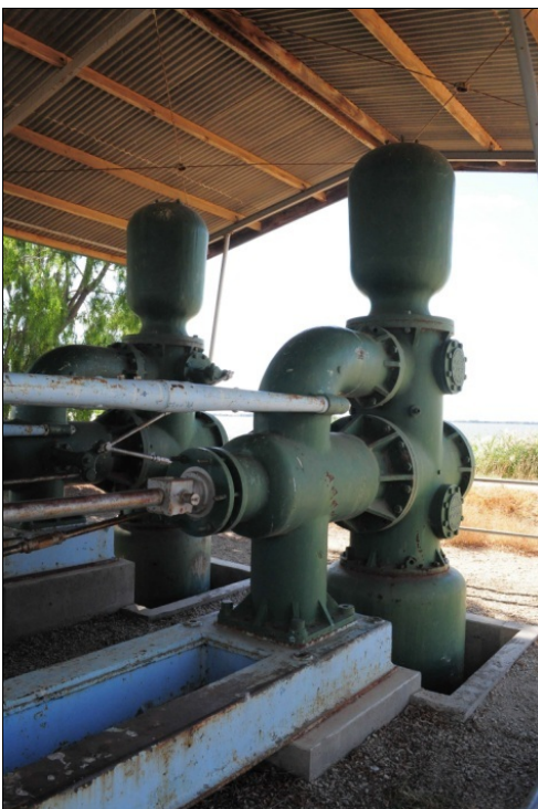
Image (left): Detail of the Cannie Ridge Engine showing the two pumps. Image: O. Peake.
