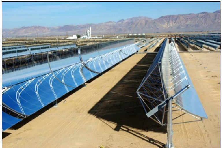
Skyfuel Trough Array.
