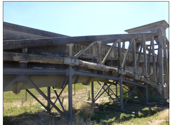
The aqueduct today, concrete spalling, propped, fenced off and disused. Photo - David Beauchamp
