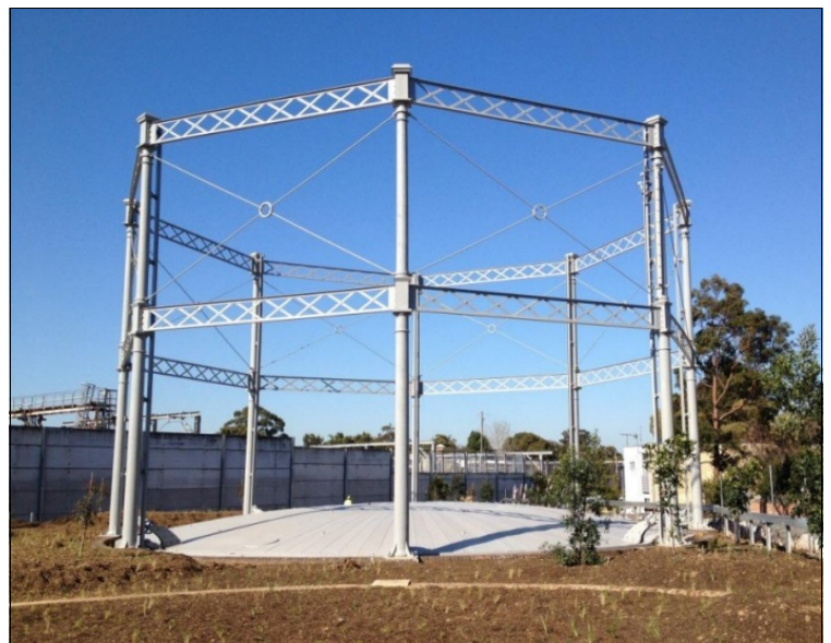
Restored Southern Gasholder at the former Eveleigh Railway Workshops Gasworks, shown before the finials were attached.
