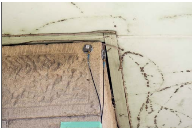
FIGURE 1 : Accelerometers mounted on the corner of a window to measure in-plane movements.
