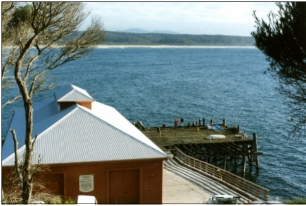
The Tathra Wharf on the South Coast of NSW – photographed partway through its restoration works in May 1985. Photo: M. Doring.
