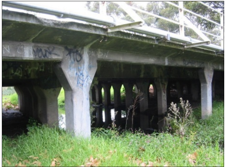
View of the St Kilda St Bridge structure from the west side. From Heritage Victoria.
