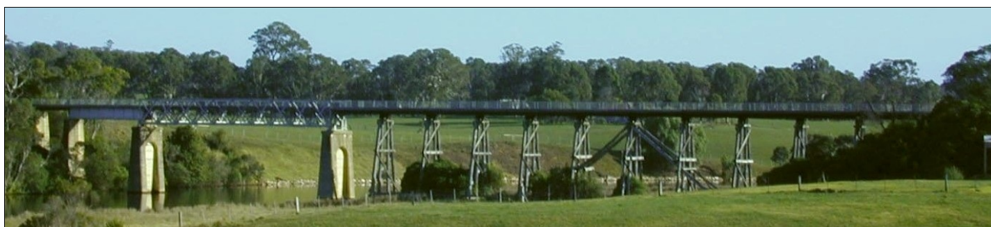
The Nicholson River Bridge as it stands today – still in use as part of the East Gippsland Rail Trail
