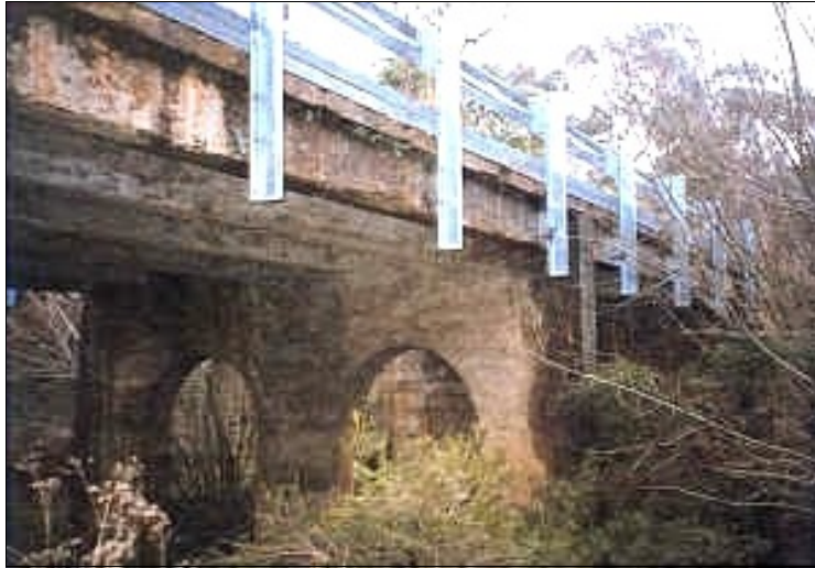
Excelsior Bridge in c1997, showing the form of the central pier. Photo Lesley Alves from the Alan Holgate website.
