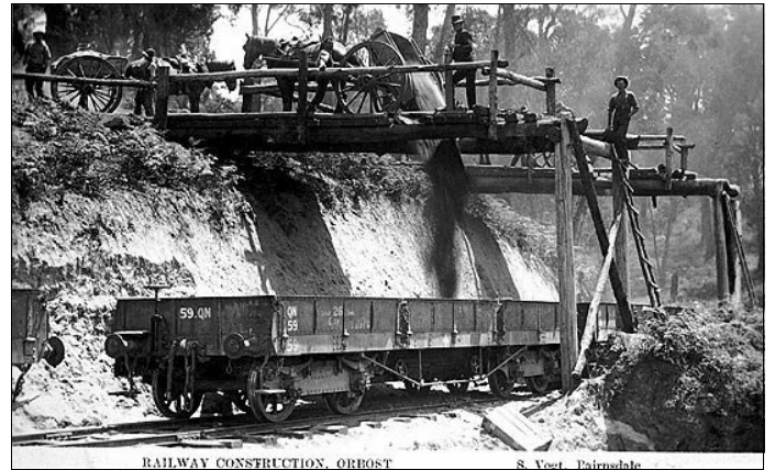
Horse-drawn tipping cart dumping fill through a timber platform into rail wagons below during railway construction 1914. Photo S Vogt, Bairnsdale
